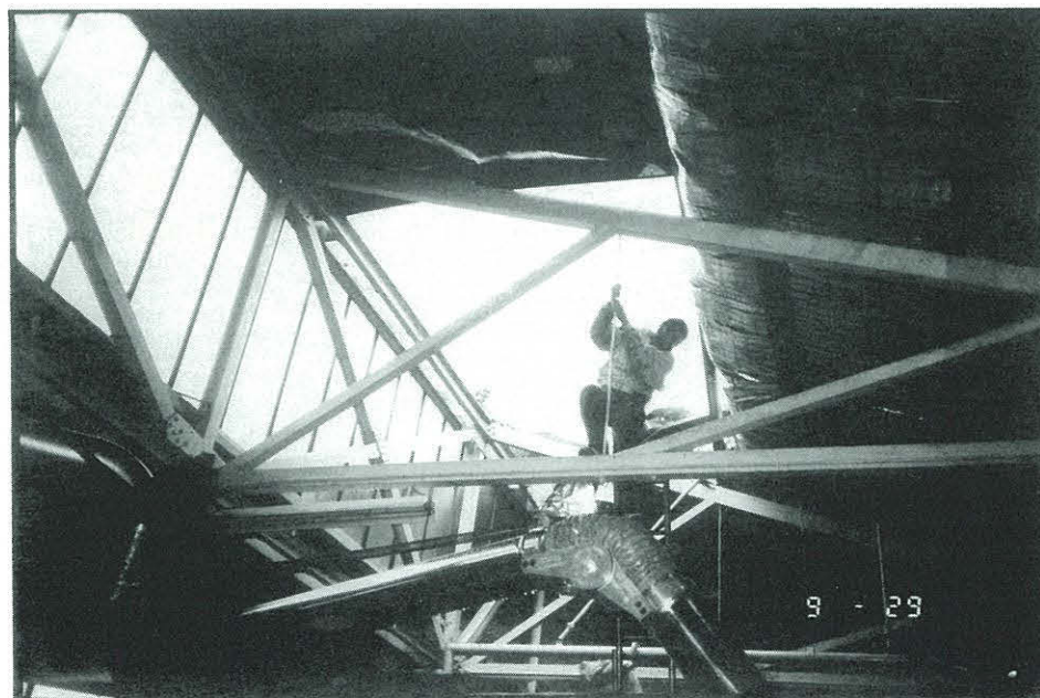
A fierce storm in August 1990 damaged the roof of the Australian National Maritime Museum's Union Street administration building. Within a couple of hours assistance had arrived and by the end of the day the building was stable and affected material had been given first-aid treatment to ensure it dried safely. Photo courtesy Australian National Maritime Museum.
